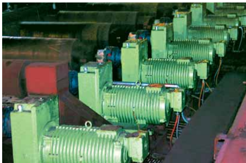
Top: VEM gearbox motor ready for shipment Bottom: Fully installed drives of the beam rolling train
