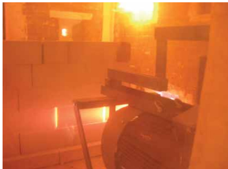
Smoke extraction motor in service
