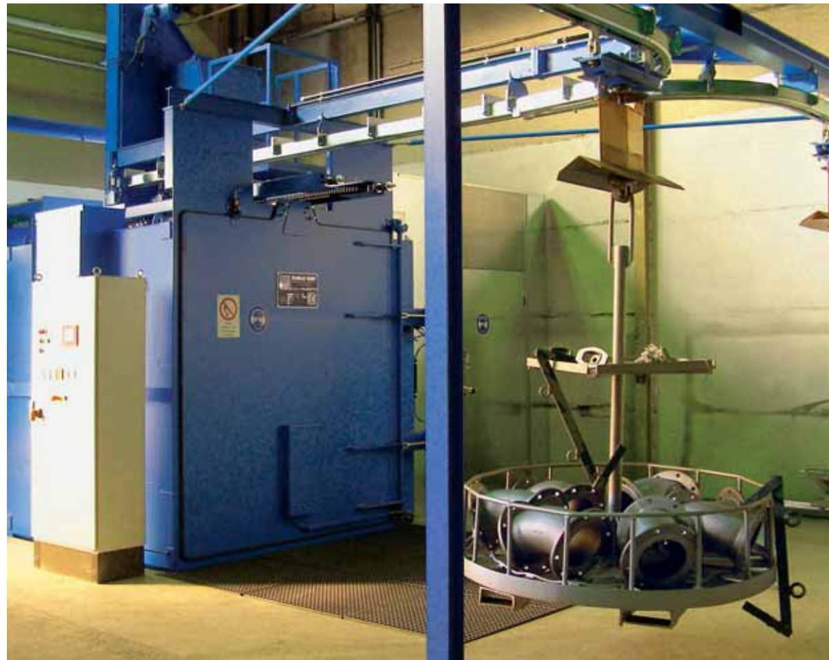
The new overhead conveyor blasting unit in Keulahütte
