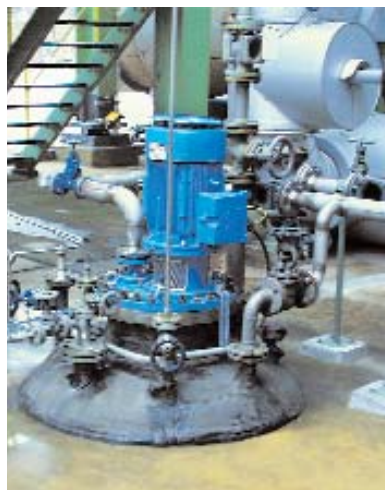
Shaft waste water pump. Explosion-protected electrical equipment is prescribed in areas in which explosive gas-air mixtures may occur.
