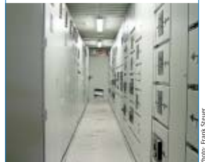
The installed load of the container switchplant amounts to 2 x 4,000 A
