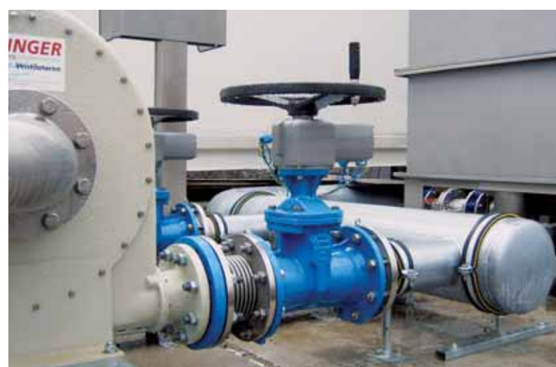
The biogas co-generation plant in Zittau is equipped with gas valves from Keulahütte.
